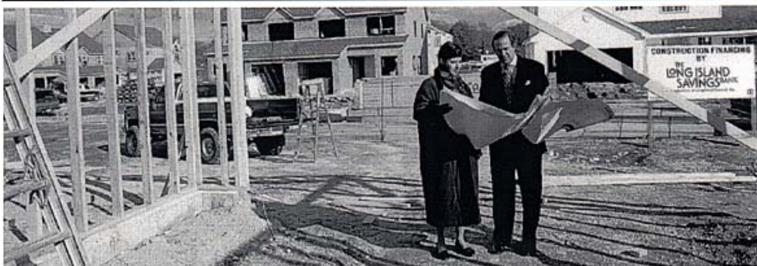
Pictured at the Villages of Huntington construction site are Susan Barbash, principal partner of McGovern-Barbash Associates of Babylon (left), and Bruce Barnet, executive vice president of real estate and development for The Long Island Savings Bank.
